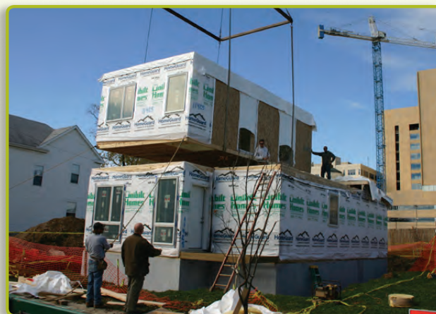
The second floor of the Litehouse is lowered in to place at 65 Frank Street in the Fairgrounds Neighborhood.
